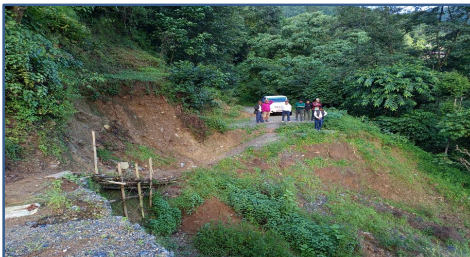
Road damage at Vedhikhor Hugdishir
