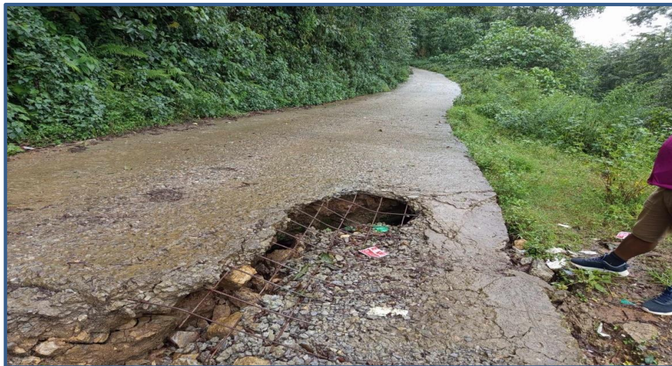
Road Damages near Satdobato
