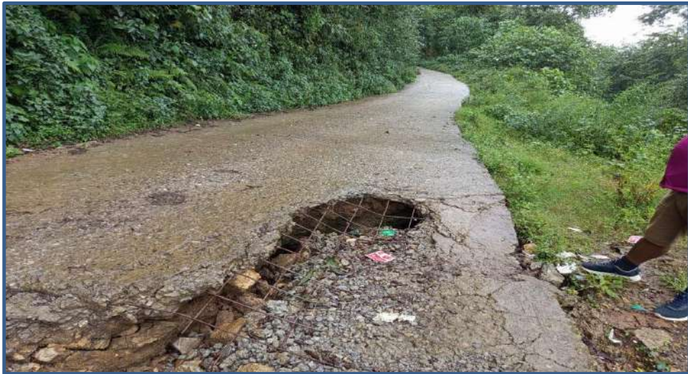
Road Damages near Satdobato
