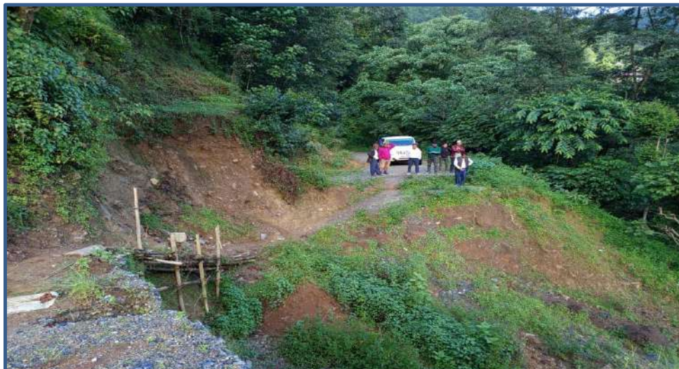
Road damage at Vedhikhori Higdishir
